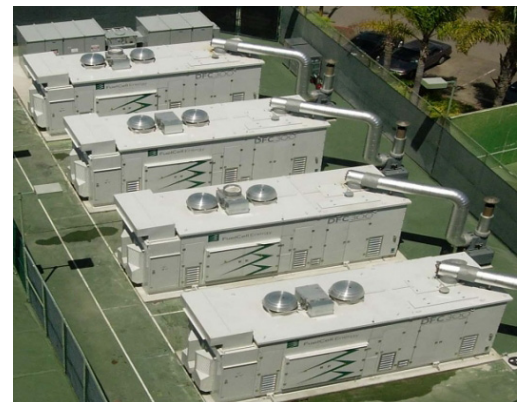
Hydrogen fuels stationary fuel cells providing primary power.
