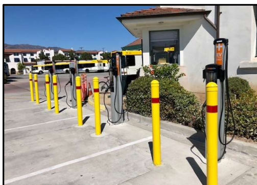
SB Metro Transit District
