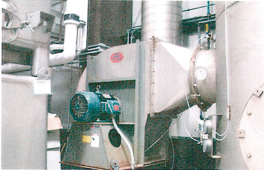
Packed bed scrubber blower
