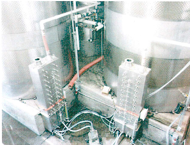
NoMoVo control systems (2)
