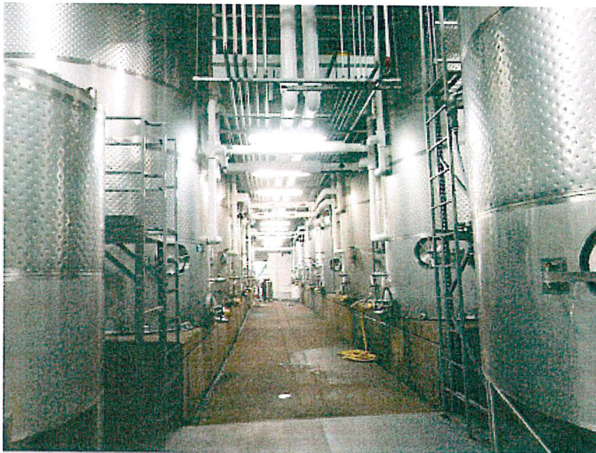
CCWS Series 400 tanks and EcoPAS piping manifold
