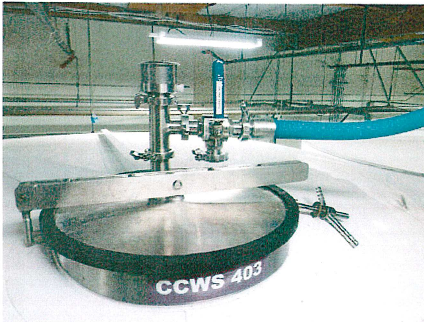
Closed top fermentation tank with EcoPAS piping
