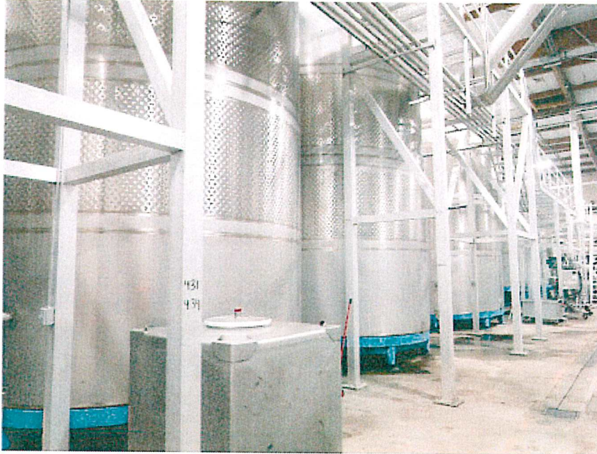
CCWS Series 400 tanks and EcoPAS piping manifold
