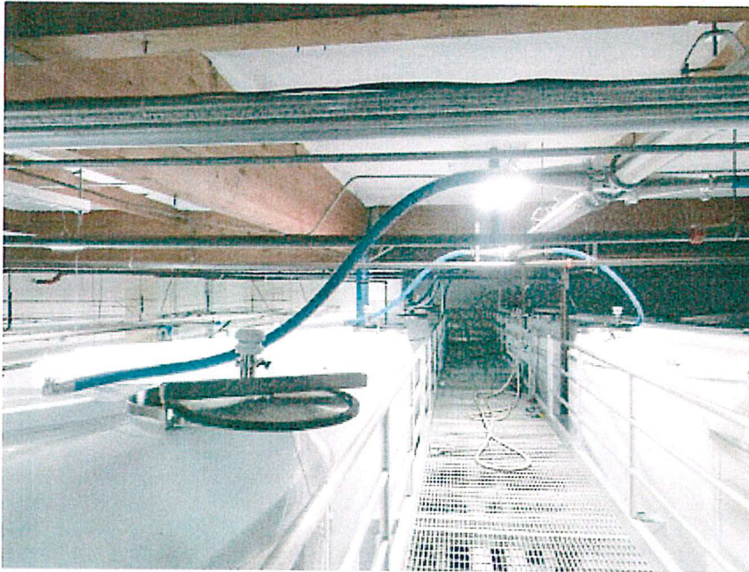
Closed top fermentation tanks with EcoPAS piping manifold
