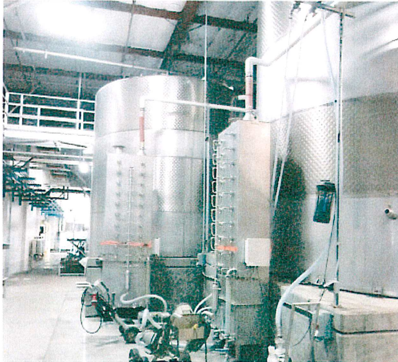
NoMoVo control systems (2)
