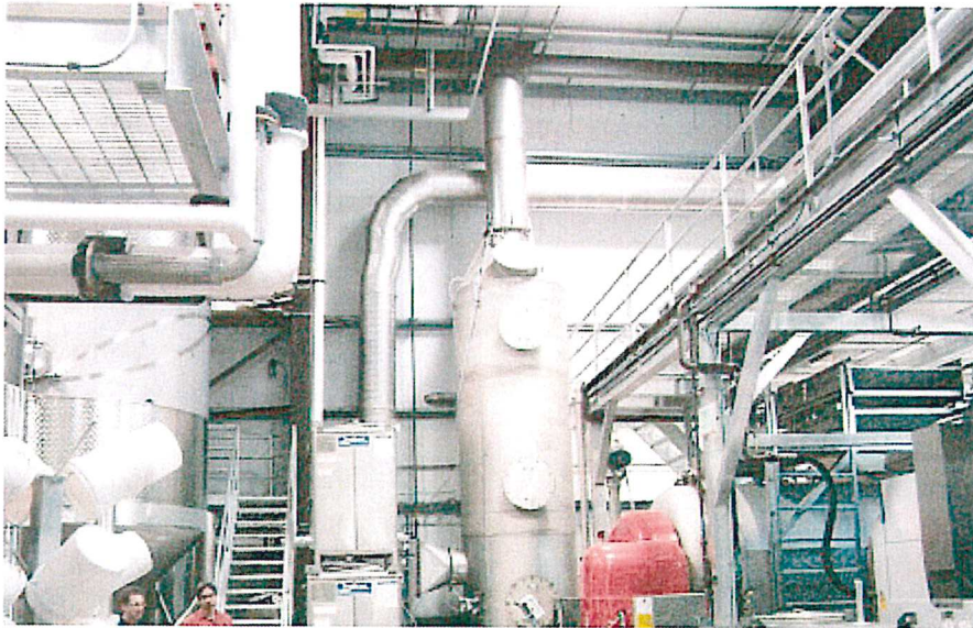
Packed bed scrubber
