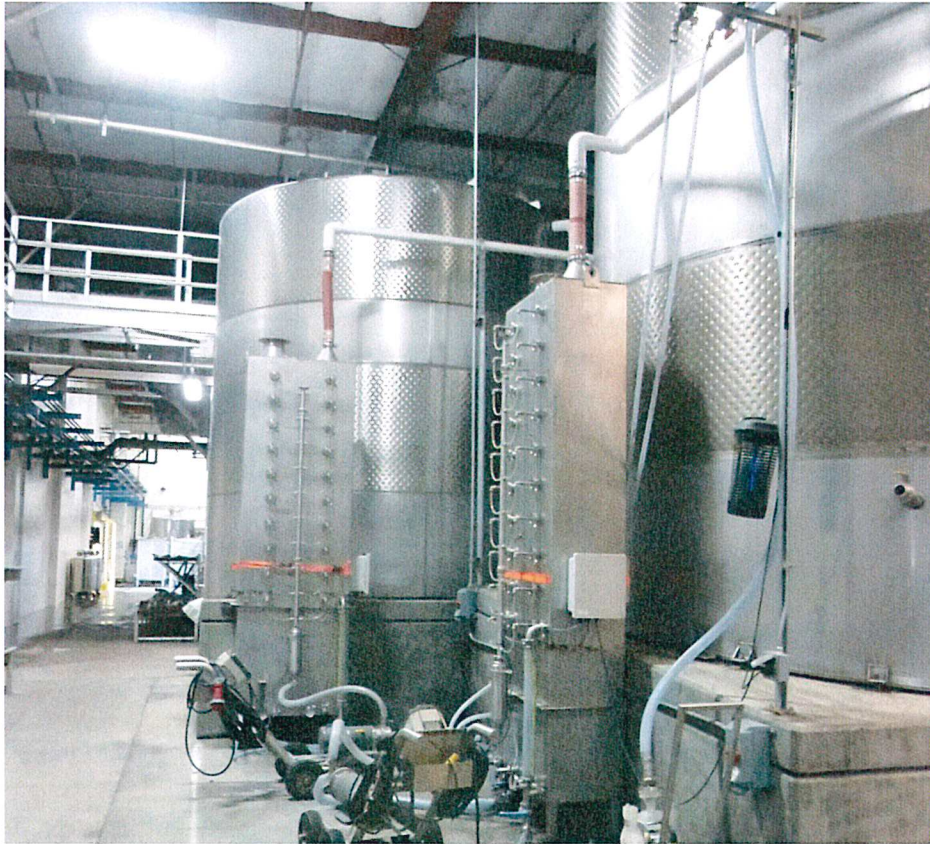
NoMoVo control systems (2)
