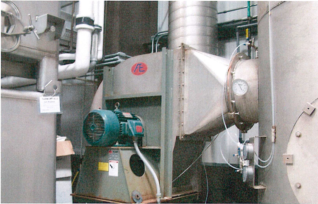
Packed bed scrubber blower
