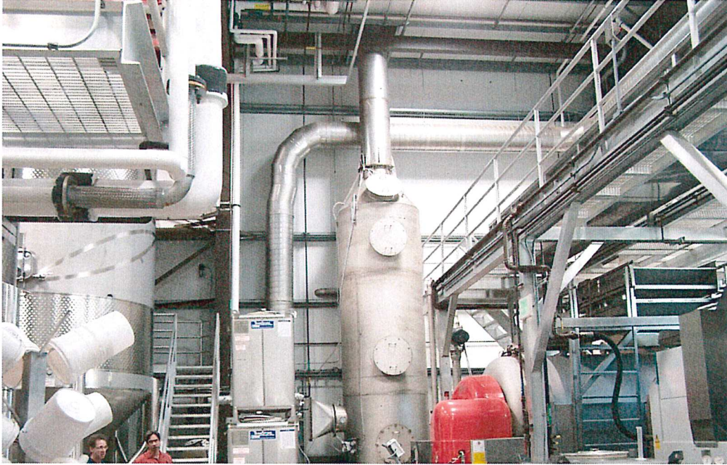
Packed bed scrubber
