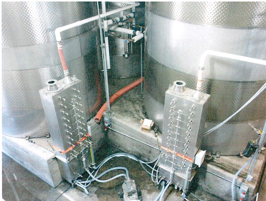
NoMoVo control systems (2)
