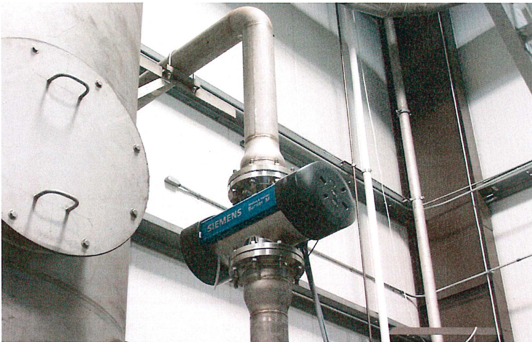
Packed bed scrubber and UV treatment lamp
