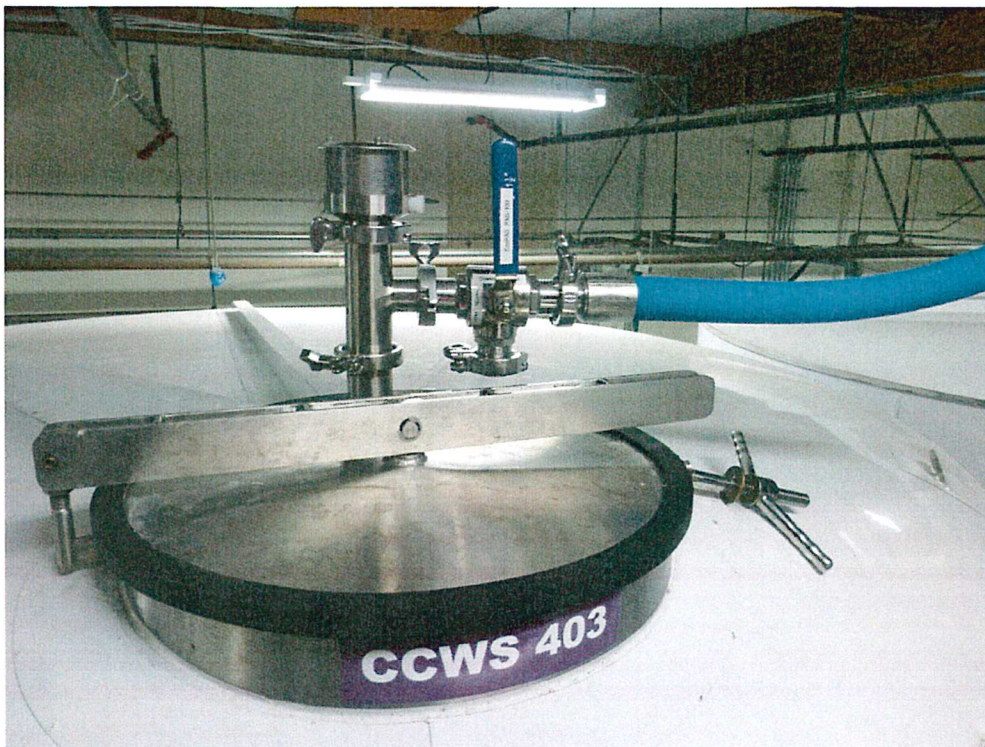
Closed top fermentation tank with EcoPAS piping
